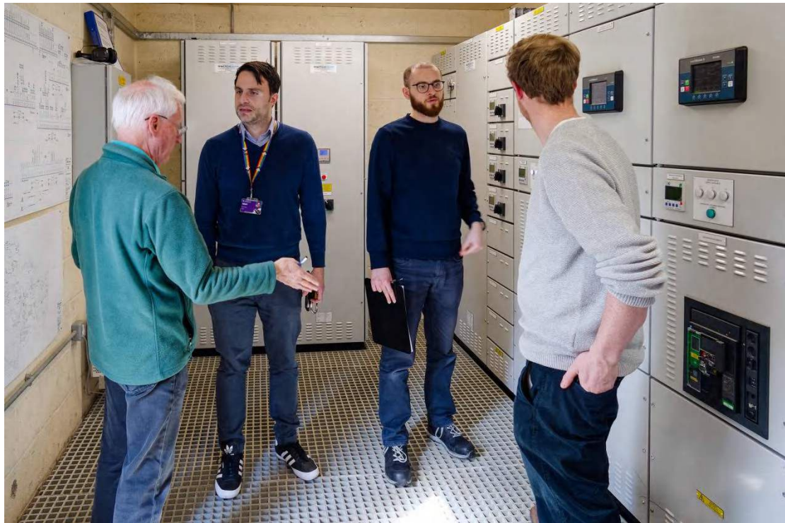
1 st site meeting for the project at Leahurst with consultants Scene Connect
